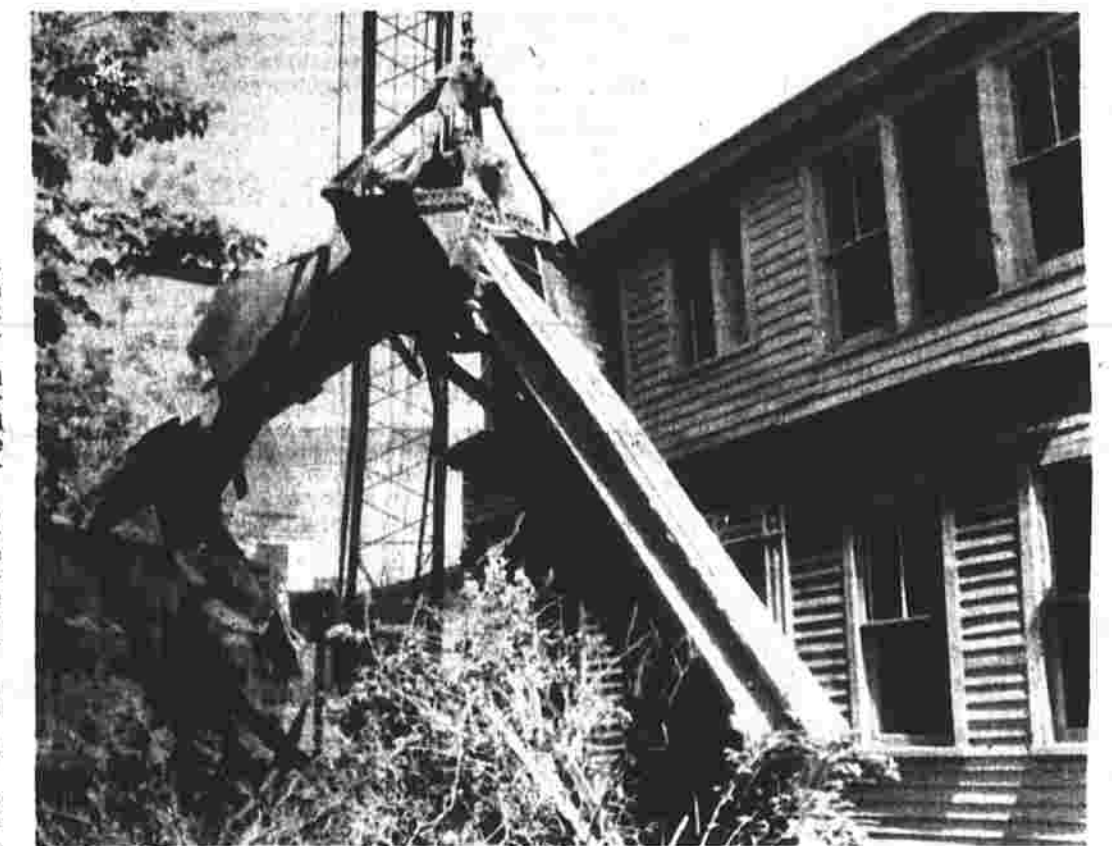
Demolition crews moved in this morning to tear down the 1827 house that served as headquarters for the Manchester Child Guidance clinic for about 17 years. Equipment of Manalorf Brothers of New Britain takes the first bite out of the front porch. Story on page 8. (Herald photo by Richmond)
